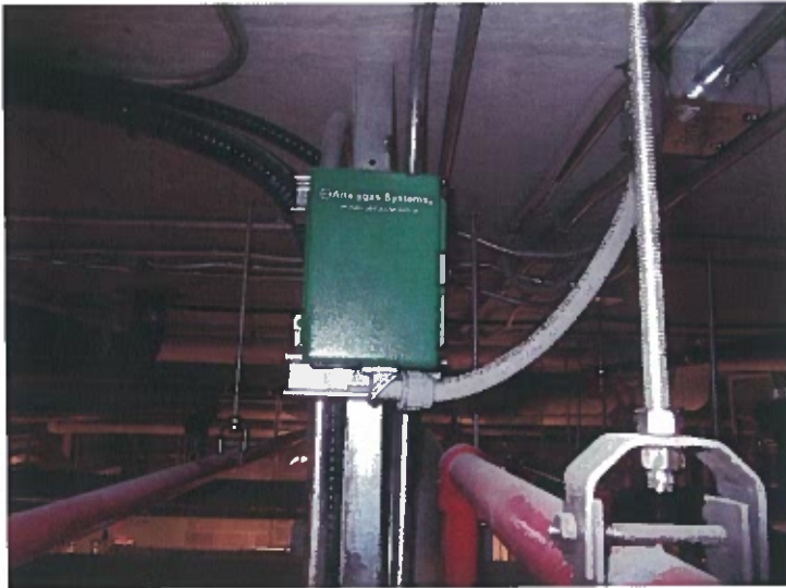
Analygas Systems Ammonia Sensor located above the North end of Compressor #2
